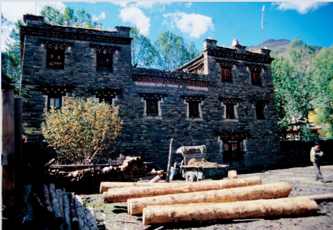
FIGURE 1 Logs being gathered for house addition. In eastern Tibet—where wood is plentiful and houses are larger than in the west—houses are often referred to by the number of columns or pillars they have. (Photo by William Semple)
